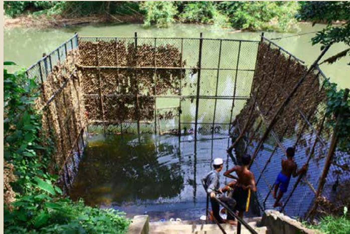
Figure 38: Accumulated debris (Type 1 CEE)
